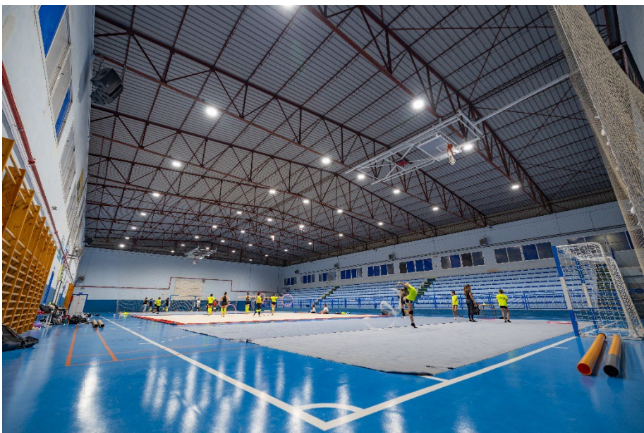
Mirella Belmonte indoor sports hall brightly illuminated with LEDVANCE LED high-bay luminaires
