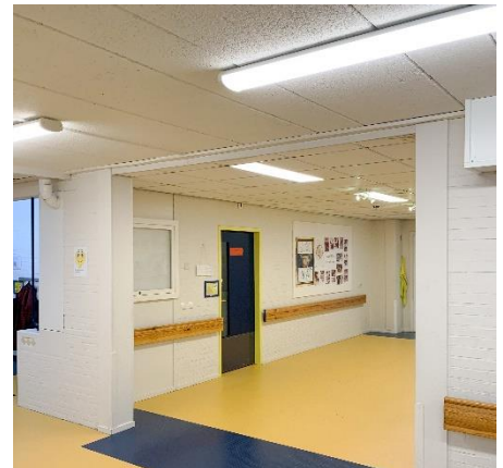
LEDVANCE LINEAR SURFACE IP44 luminaires as well as PANEL 1200 luminaires have been installed in the school corridors.
